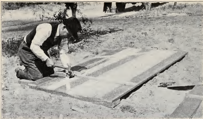
Fig. 8—Nail the 1×2-inch baffle cleats firmly in position after trimming the side-wall sheathing.
